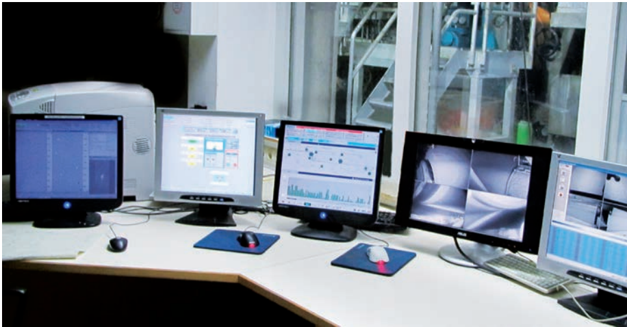
Figure 4: The machine control room also provides access to information about the current state of the PROFIBUS network via the PROFIBUS Monitor.
