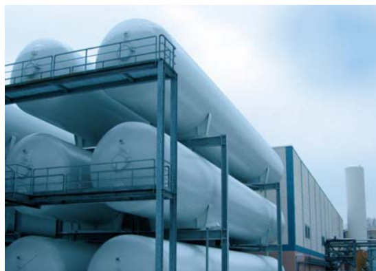
Cooling plant with helium reservoirs
