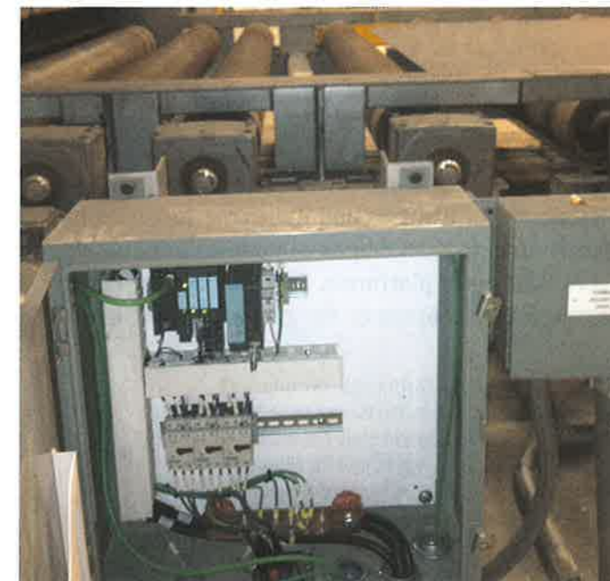
Individual PROFINET field devices are installed onsite. The open motor control cabinet shown here is used for decentralized acquisition of different motor signals.
